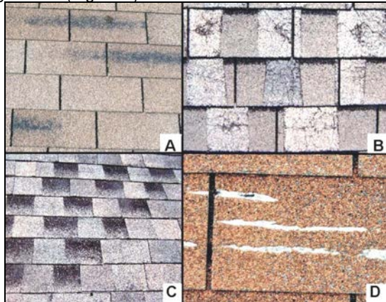
Figure 5. Various shingle manufacturing defects: a) lack of granule adhesion on a three-tab, b) blotchy appliques, c) asphalt exposed in lower laminate, and d) lines of missing asphalt and granules.
