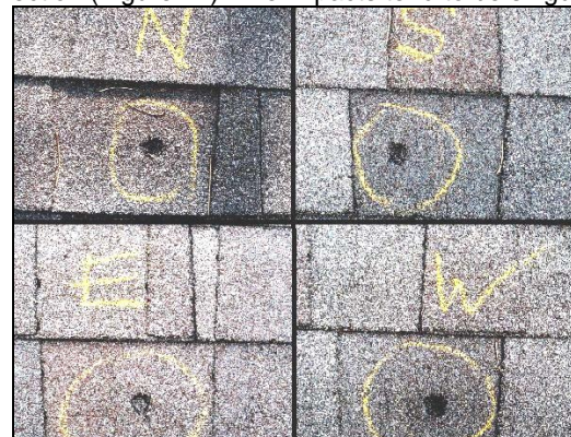
Figure 11. Attempts to simulate hail damage with a ball peen hammer.
