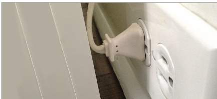
Within electrical cords accidentally damaged by furniture resting or pressing upon them
